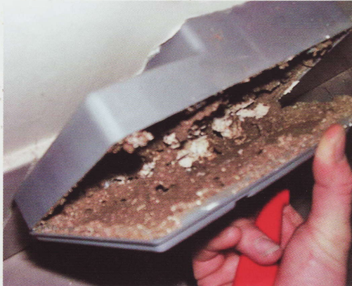
Above ground station with termite activity.
