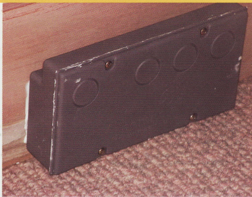
Above ground station placed on damaged wall.
